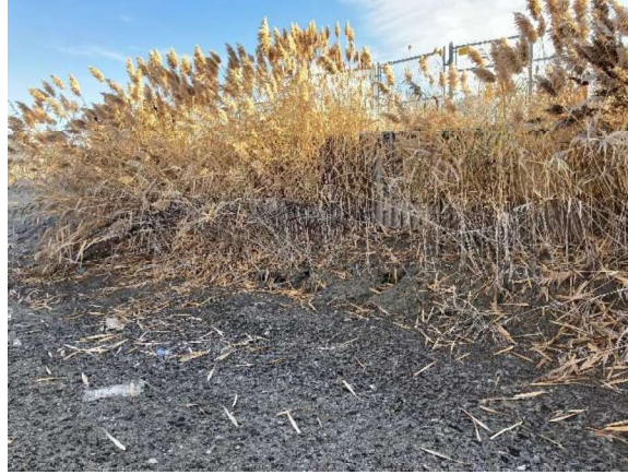
Photo 2-12: Excessive Vegetation Blocking the Storm Water Dumpout on USLC to Midas Creek
