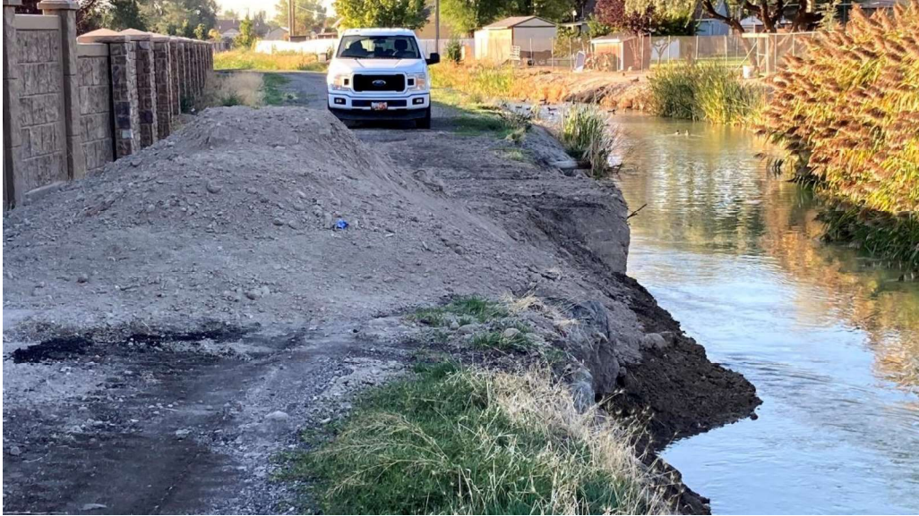
Photo 2-7: Recently Sloughed South Jordan Canal
