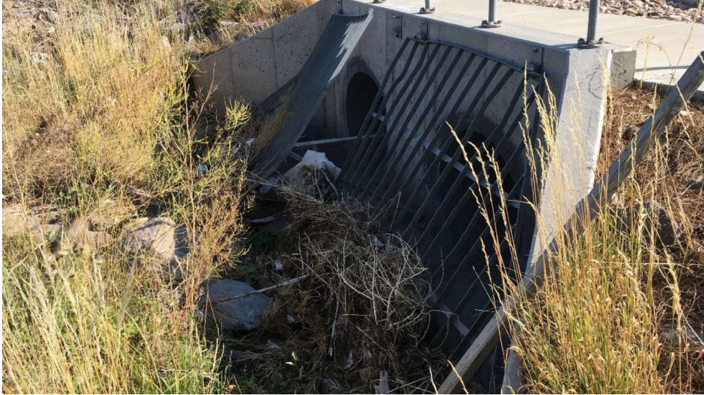
Photo 2-6: Example of a Trash Rack on Barneys Creek at Airport Rd
