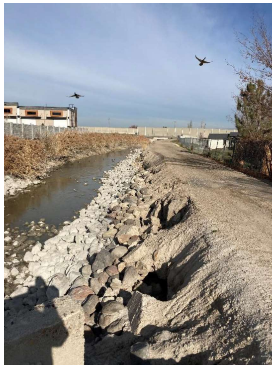
Photo 2-8: Example of Eroded Bank along Utah and Salt Lake Canal
